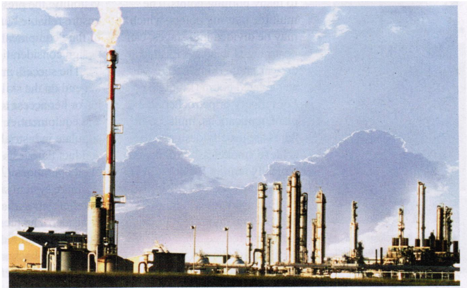
▲ Figure 1. Typical elevated single-point flares fire upward.
